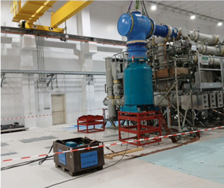
Figure 29: Hi-pot Test kit installed on Bus Section A, Red Phase
