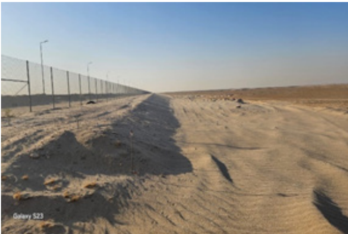
Slope Preparation in West side of MEG Pond Area - for Polymer Spray
